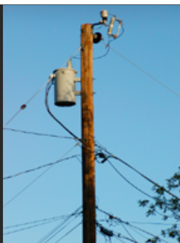
Utility pole tube holding utility tubes and transformers as distributed centers.
